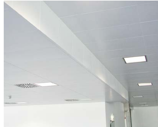
clean-ceil grid panel ceiling with step in the ceiling
